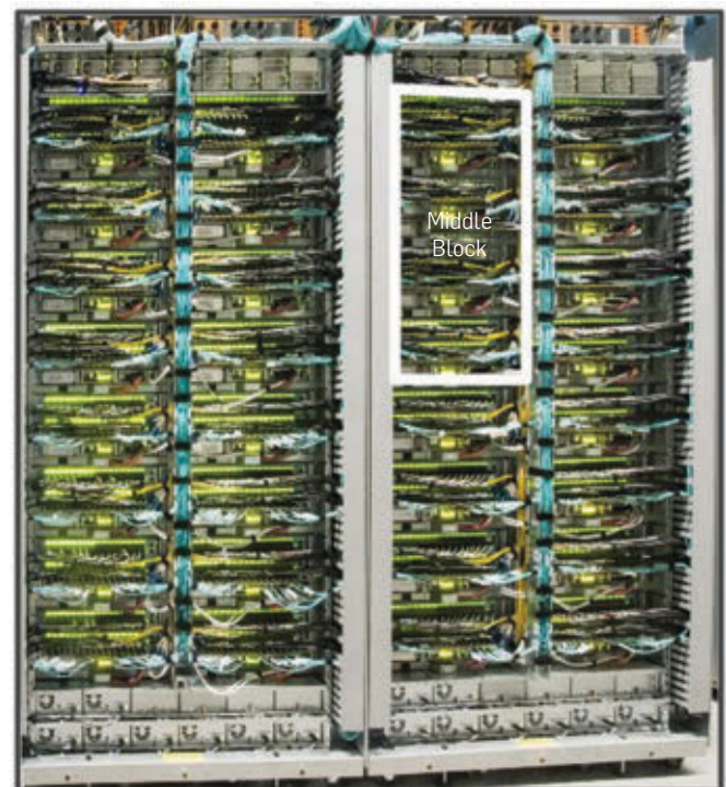
Figure 9. Jupiter Middle blocks housed in racks.
